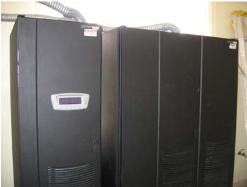
Larger system wide UPS systems are another option when grid outages are short and/or a back-up generator is available.
